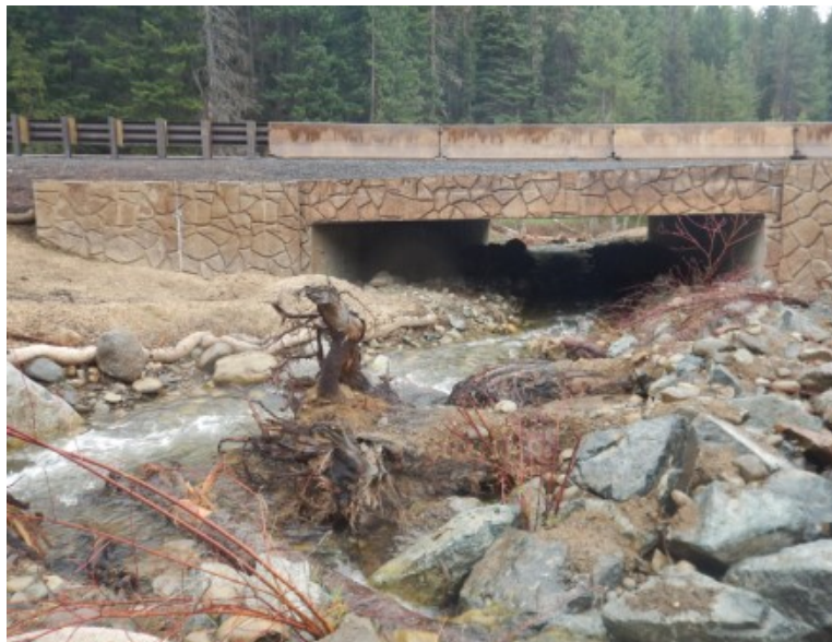
SSB 5381 clarifies the permit process for fish passage projects. Photo: WSDOT improved culvert on Swauk Creek, I-97
