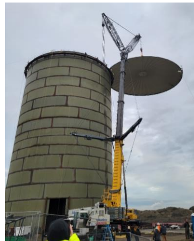
Photo credit: City of Pasco, Zone 3 Reservoir Storage Tank
